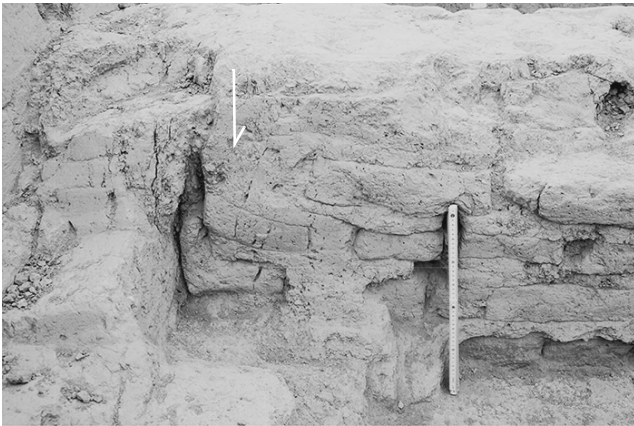
Fig. 16. Subsidence of the main wall at f.s. 4 (Fig. 10) is indicated by white arrow. Due to the subsidence, the clay bricks at the junction with the opposite wall are curved downward. Cracking of both walls at their junction is noted.
